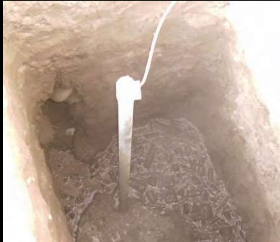
GI pipe to connect plate to the earth surface
