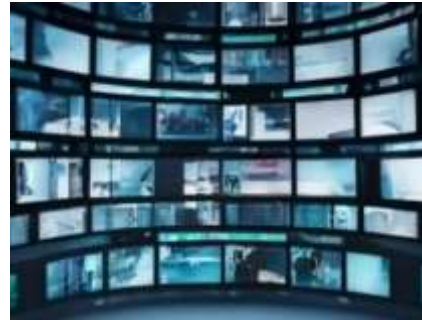
Figure 1.2: CCTV Video Monitors
