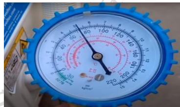
Fig. 2.69 Pressure value in the pressure gauge
