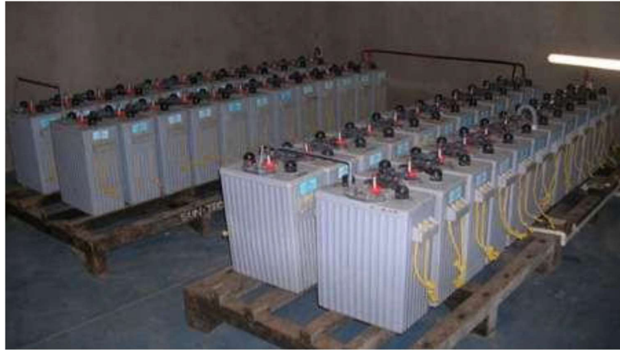
Fig. 9.5: Location of batteries in a well-ventilated room
