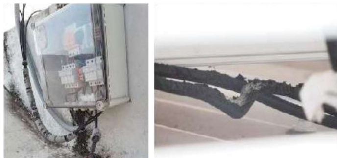
Fig. 9.9: Poor quality conduit and unprotected cable can be easily damaged
