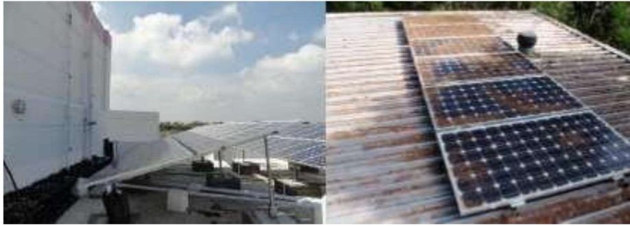
Fig. 9.2: Incorrect site selection for array installation
