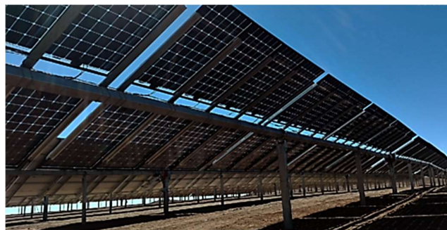
Fig. 5.6: Bifacial Solar PV Panel
