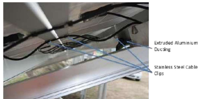
Fig. 9.8: Properly managed PV array cable
