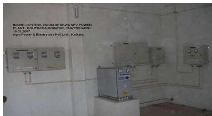
Fig. 9.4: Inverter and control equipment installed in a control room
