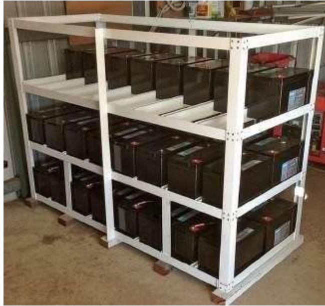
Fig. 8.22: Battery Bank enclosures/racks
