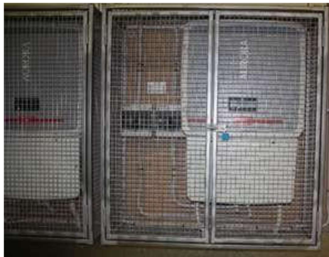
Fig. 9.3 Access to the inverter is controlled
