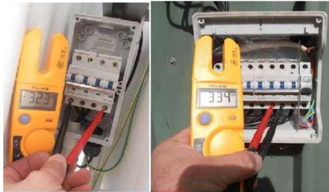
Fig. 9.11: Checking of reverse polarity using a clamp-on meter (Voltmeter)
