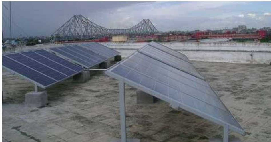
Fig. 9.1: Shadow-free installation on Howrah Municipal Corporation Building
