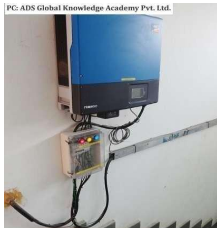
Fig. 8.28: Inverter and AC distribution box
