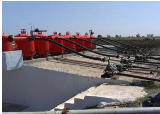
Figure 1.3: A series of filters installed for a drip irrigation
