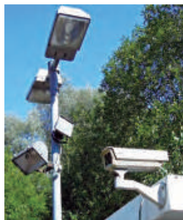
Fig. 3.9: Security lighting system with CCTV camera
